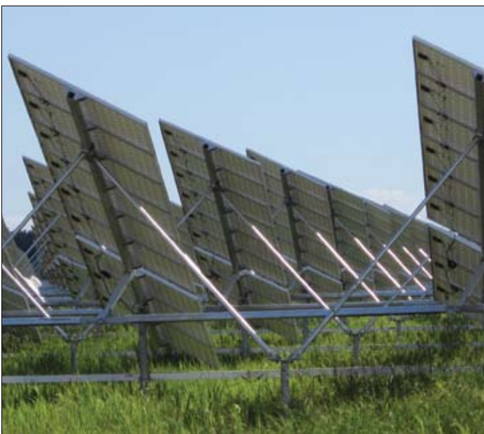
The photovoltaic panels at the Amherstburg facility are computer controlled to follow the sun.
