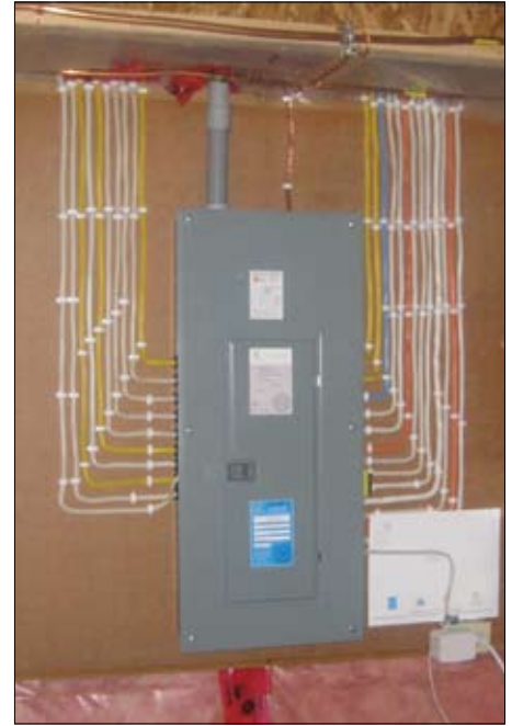
Copper power and communications wiring for the automated, energy efficient home. The pride in Gilles Michaud's quality homes is clearly evident.
