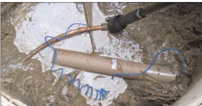
The completed replacement at the curb stop includes a 5.5 kg (12 lb) sacrificial zinc anode.
