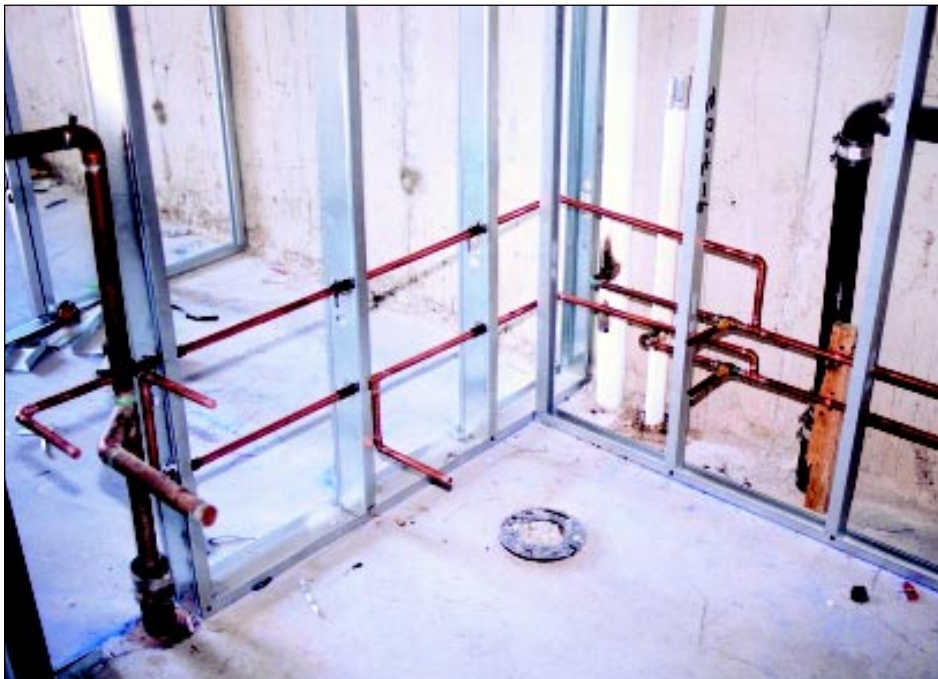
Neat copper drainage, vent and water supply lines in a modern condo bathroom.
