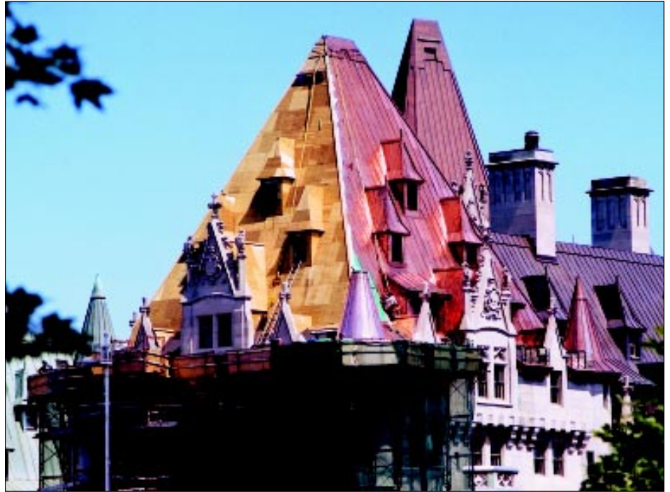
The installation stages from the plywood substrate to the copper sheet can be seen in this section of the roof.
