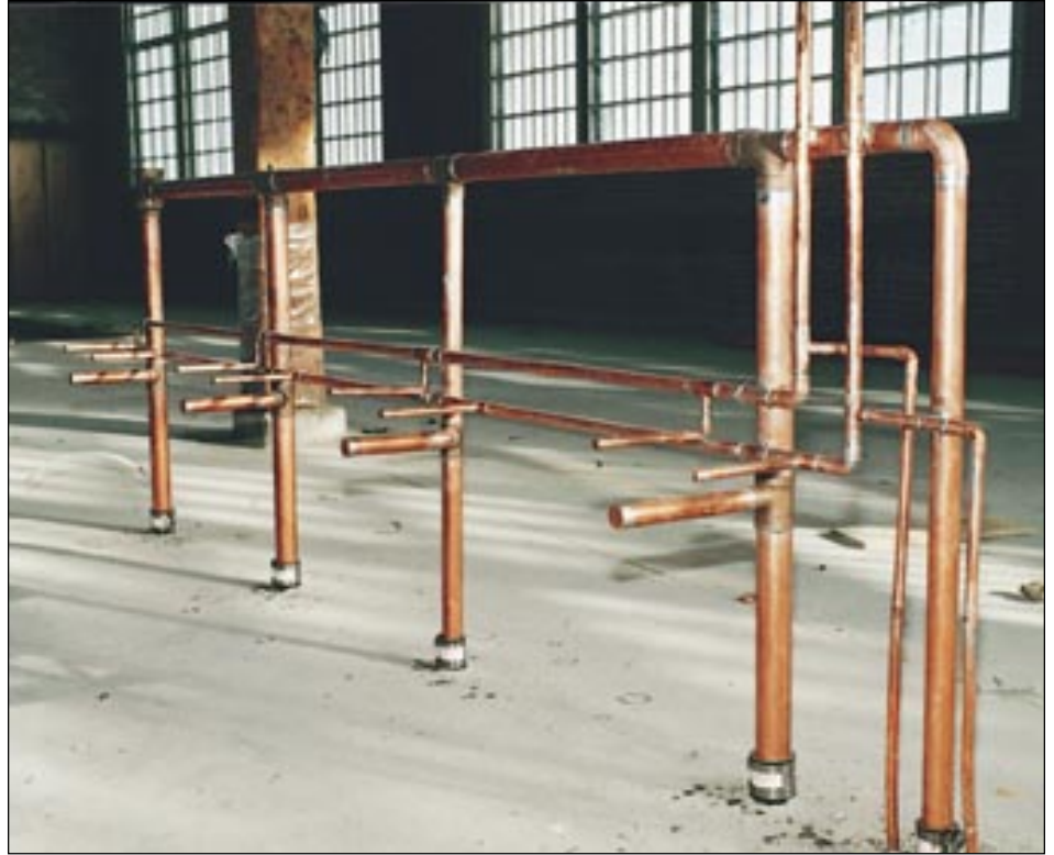
The quality of workmanship is evident in the plumbing for this bank of lavatories.
