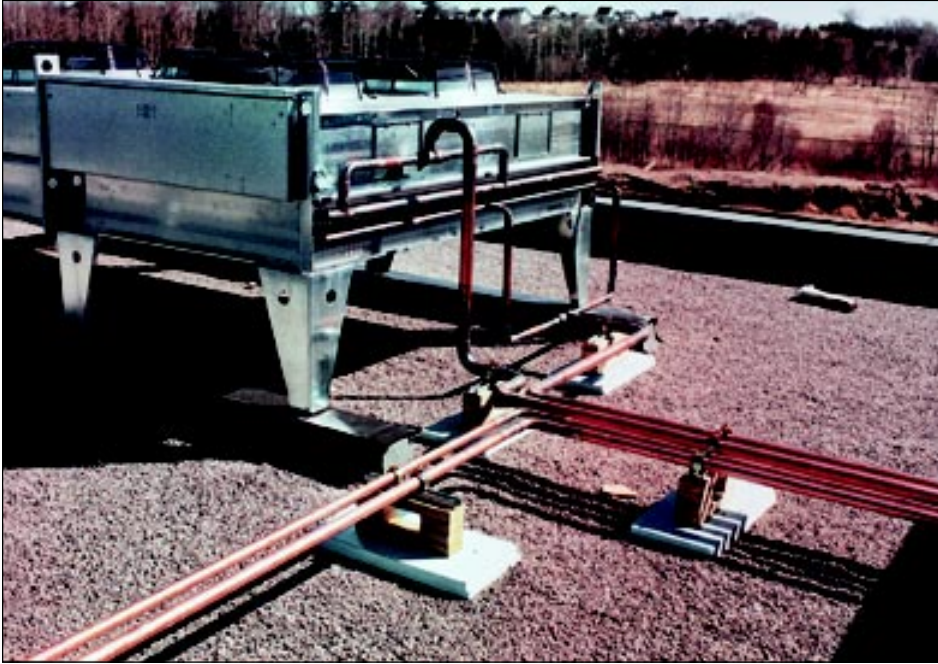
The roof mounted fan coil heat exchangers are connected to the refrigeration system by runs of copper tube.
