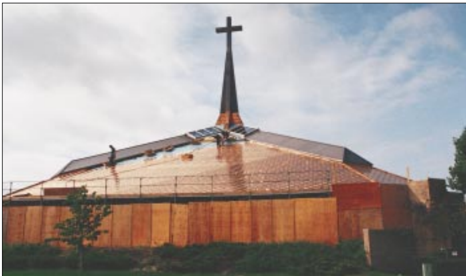
St. Justin's Church, with the newly installed flat seam spire and CastleTop Metal Tile roof.
